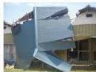
Photo 3: Impact from flying debris (roof)
