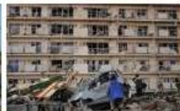
Photo 5: An apartment building with extensive damage to non-structural elements
