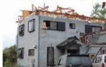
Photo 2: Destruction caused to a wooden house
