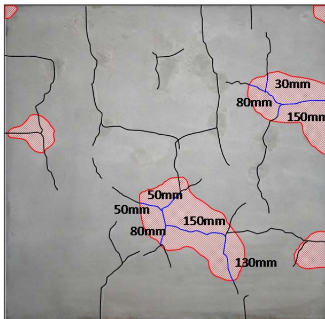
図-3.2.28 No. 6 浮き・ひび割れ発生状況[E3-A]
