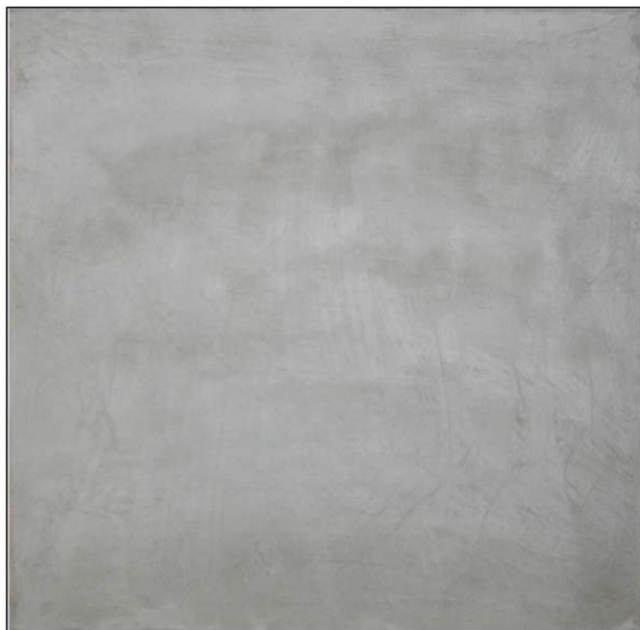
図-3.2.30 No.8 浮き・ひび割れ発生状況[E3-C]
