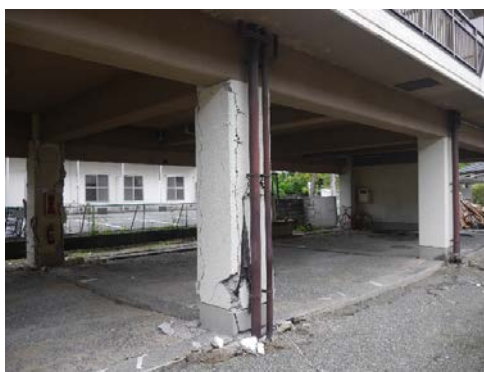
写真5.5-14 X3-Y1 柱 (付着割裂破壊、損傷度IV)
