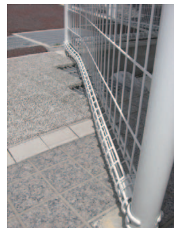
(c) 侵入防止柵のゆがみ
