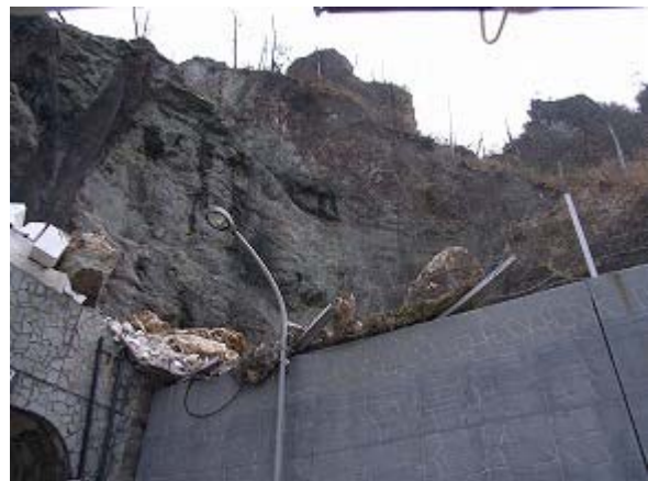
2-f 崩落面遠景
