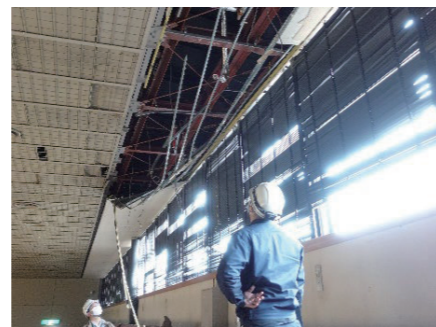
福島県沖を震源とする地震による建築物等被害現地調査 On-site survey of damage to buildings caused by the earthquake off the coast of Fukushima Prefecture
