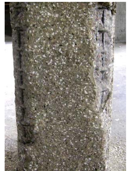
Photo 5: Spalling in concrete components
