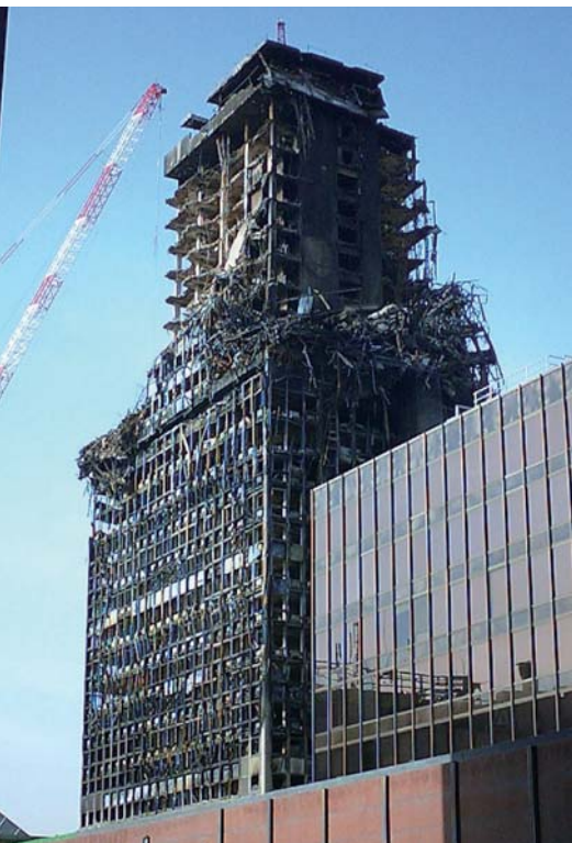
Photo 1: Total destruction of high-rise building in Spain with large-scale collapse of the upper floors
