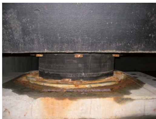
Photo 9.2-10 Rust of High-damping rubber bearing
