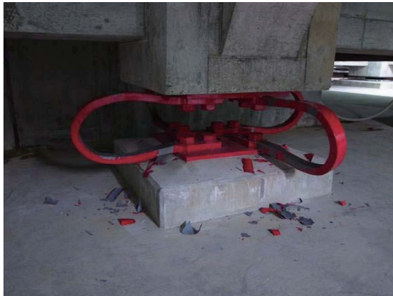
(a) Peeling off of paint
