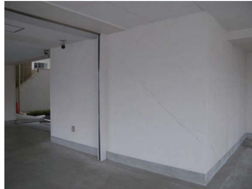
Photo 9.2-14 Shear crack on the wall
