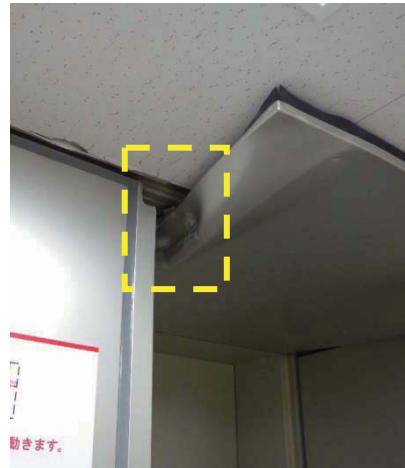
(b) Damage to the expansion joint
