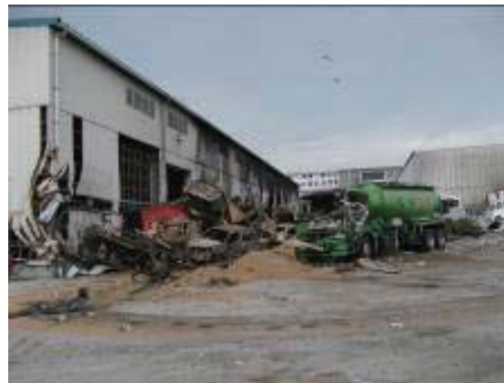
Photo 8.2-2 Tsunami fire at a port warehouse (Sendai city, Miyagi prefecture)
