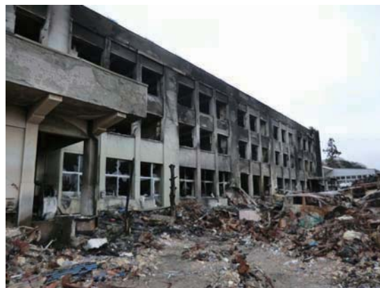
Photo 8.2-1 Tsunami fire at an elementary school (Ishinomaki city, Miyagi prefecture)
