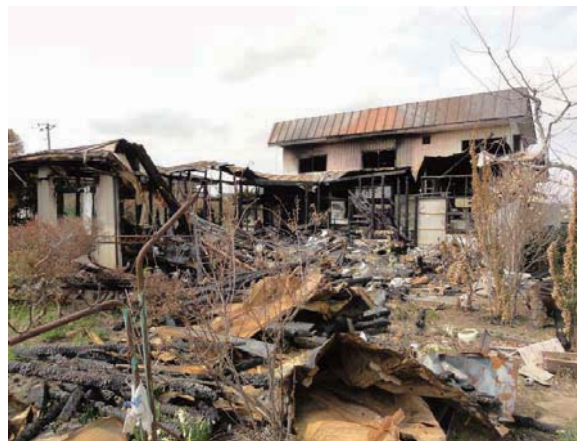
Photo 8.3-3 Fire scene at a house (Oushu city, Iwate prefecture)
