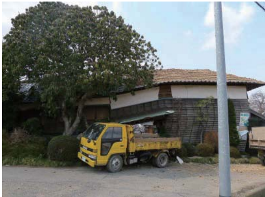
Photo 6.2-81 Heavily damaged Nagayamon gate (Yoshinuma-cho)
