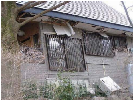
Photo 6.2-61 Failed ceiling of eave
