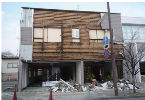
Photo 6.2-44 Fallen mortar of wall (Wood house with store)
