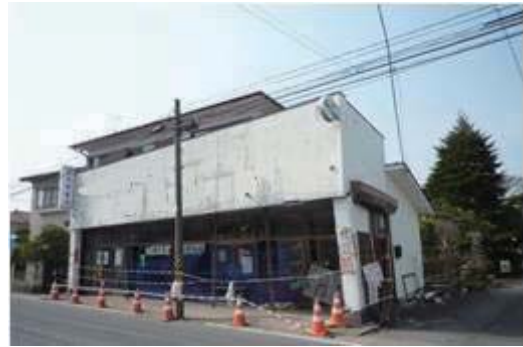
Photo 6.2-20 House with store with large story deformation
