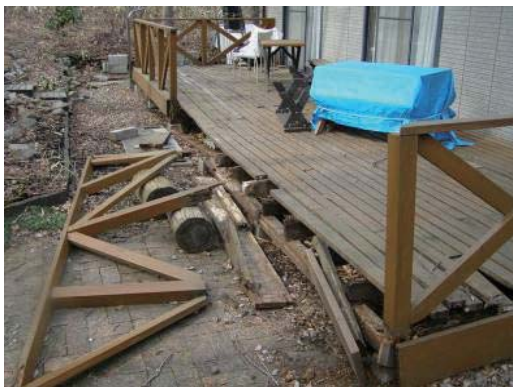
Photo 6.2-57 Damage of wood deck in Toyohara-Otsu, Nasu town
