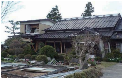
Photo 6.2-23 Largely tilted house
