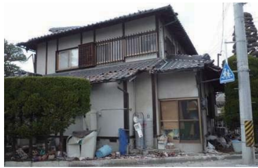
Photo 6.2-49 Damage of roof tile
