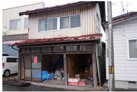
Photo 6.2-4 Damage of houses with store
