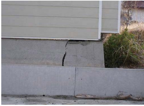
Photo 6.2-67 Crack of foundation
