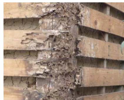
Photo 6.2-45 Deterioration and damage due to termite on column and wood lath of exterior mortar
