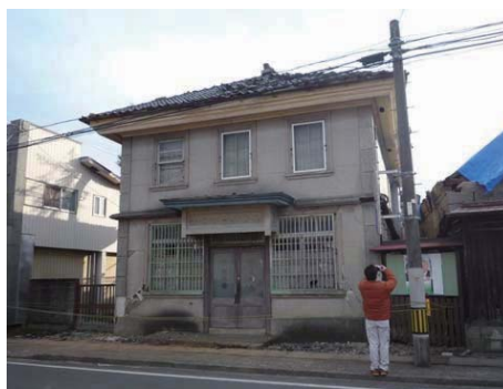
Photo 6.2-56 Damage of an old post office
