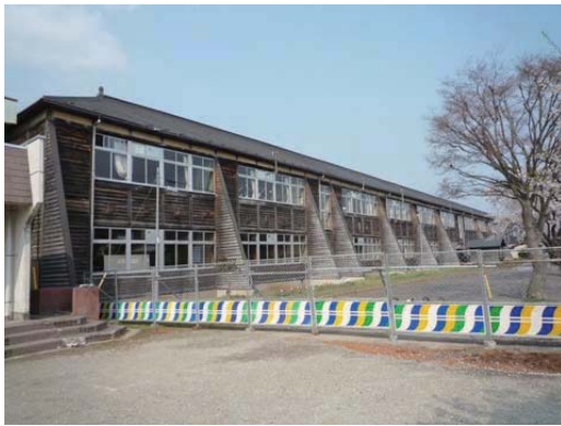
Photo 6.2-19 Seemingly slightly damaged School building
