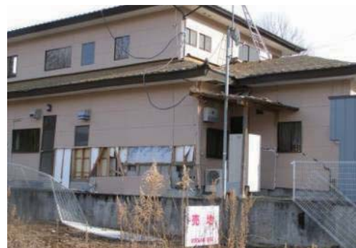
Photo 6.2-64 Damaged house due to deformation of residential land
