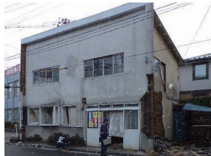
Photo 6.2-40 Drop off the mortar wall (Komatsujima)
