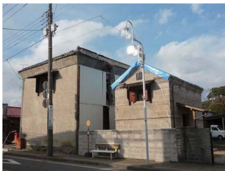
Photo 6.2-55 Damage of stone-built warehouses
