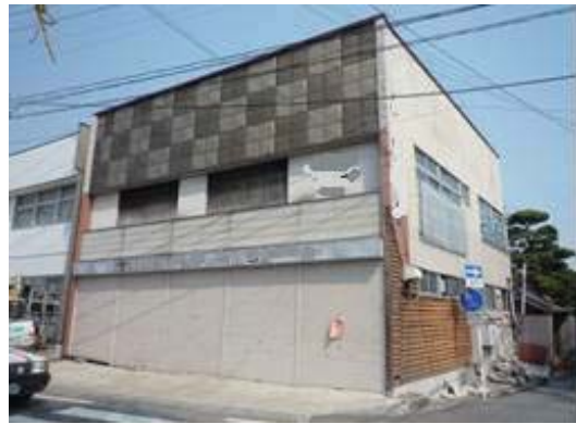
Photo 6.2-14 House with store with large story deformation
