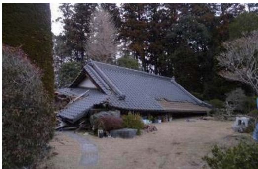
Photo 6.2-69 Collapsed wood house
