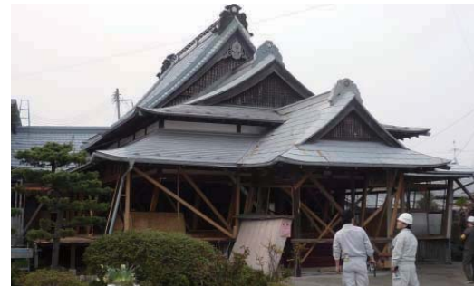
Photo 6.2-22 Heavily damaged temple building
