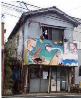
Photo 6.2-41 House with large residual deformation (Komatsujima)
