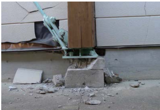
Photo 6.2-78 Breakage of the foundation concrete
