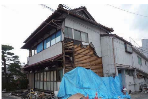
Photo 6.2-46 Collapsed stair hall
