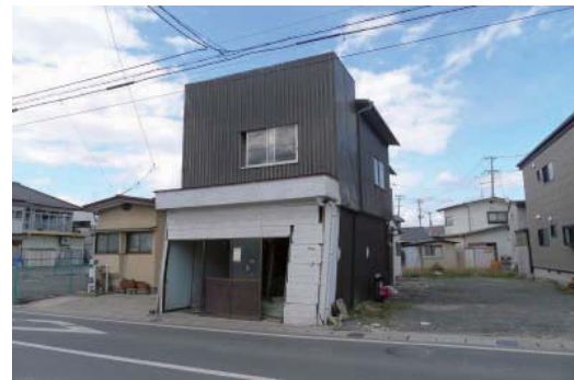
Photo 6.2-36 Tilted wood house with store
