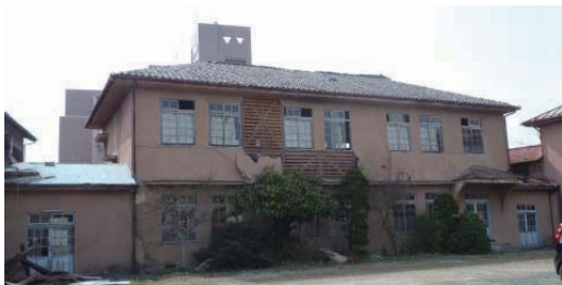
Photo 6.2-17 School building suffering damage on roof tiles and exterior walls
