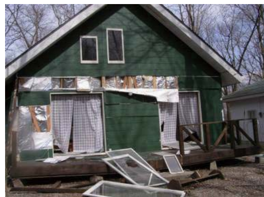
Photo 6.2-58 Heavily damaged wood house
