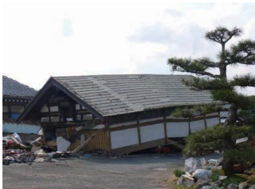
Photo 6.2-72 Collapsed nagayamon gate (Kadobe)
