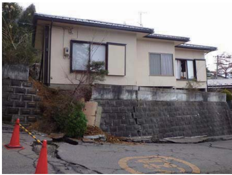
Photo 6.2-37 Damage of retaining wall and houses (Oritate, Aoba ward)
