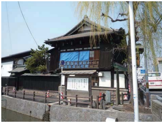
Photo 6.2-13 Damaged Japanese traditional house with large story deformation
