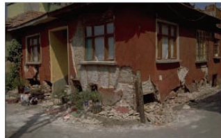
Old style CM masonry house, where wood reinforcement divides the masonry wall into small pockets which dissipate energy without leading to complete collapse after Izmit Earthquake (1999), M = 7.4.
