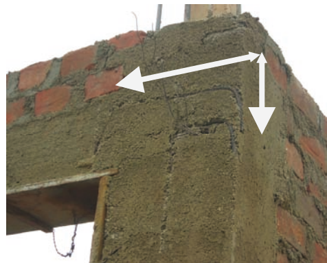
Photo.15. Lack of covering for steel reinforcement and Lack of beam's steel anchorage to the columns in Caral
