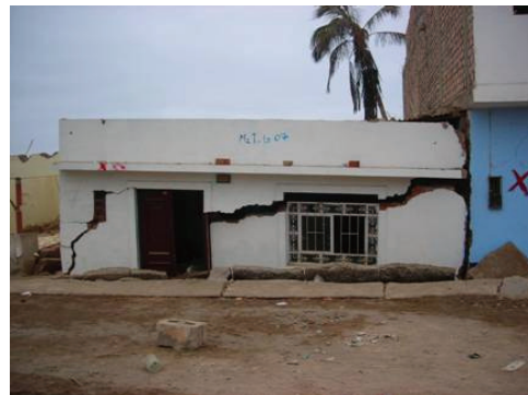
Photo.1 Damage of Near Coast of Central Peru Earthquake of August. 2007
