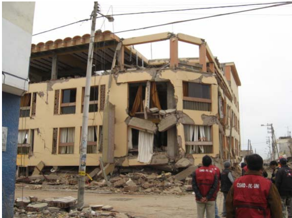
Photo 7: Damage of Hotel
