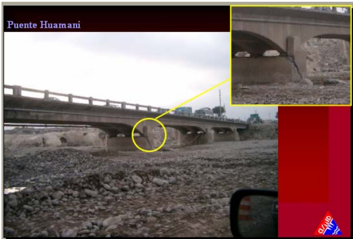
Photo 5: Damaged bridge near Pisco. It was used for a one way passage
