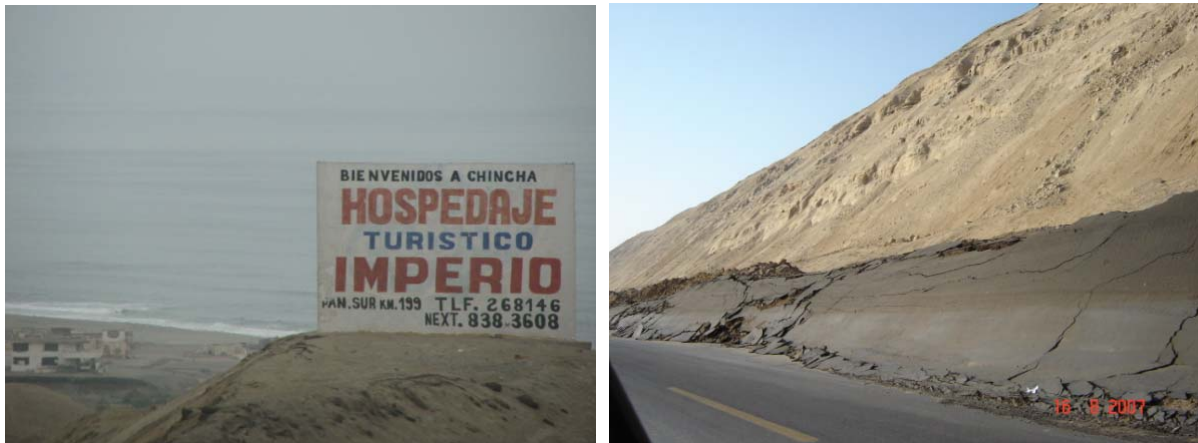
Photo 1: A part of high way was pushed up due to upheaval of east side of highway
